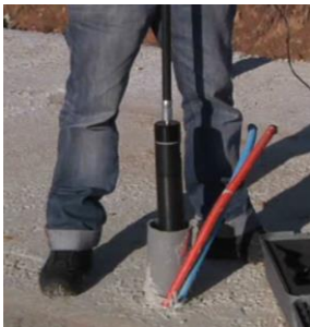
ARTHRON CAM in action investigating the condition of a vertical pipe, using guidance pole (optional attachment)
